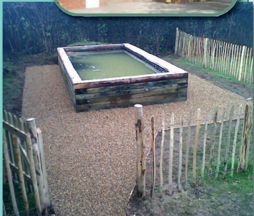
Parkers supplied timber, fixings, shingle and hardwood sleepers which formed the main structure around the top of the pond
